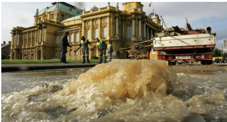
Figure 6. Water pipe perforated during survey activities for underground garage in Zagreb city centre – October 2010
