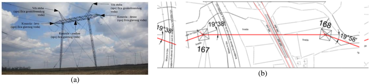
Figure 6. Powerlines (a) photo of a pole with powerlines; (b) 2D representation of powerlines
