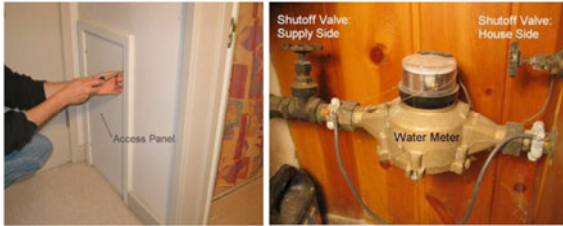
Fig. 5 Shut off valve located in access panel inside wall
